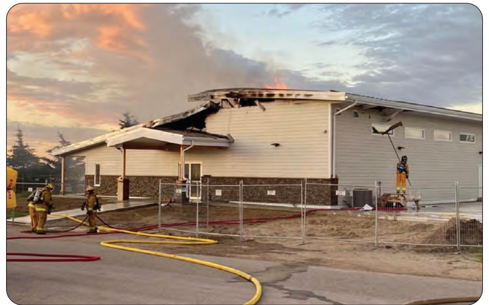
Fire broke out at the Miami Active Living Centre shortly before 5 a.m. last Tuesday.
